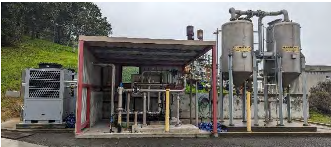
Figure 2: New Chillers and Heat Exchanger at the Biogas Treatment Area
