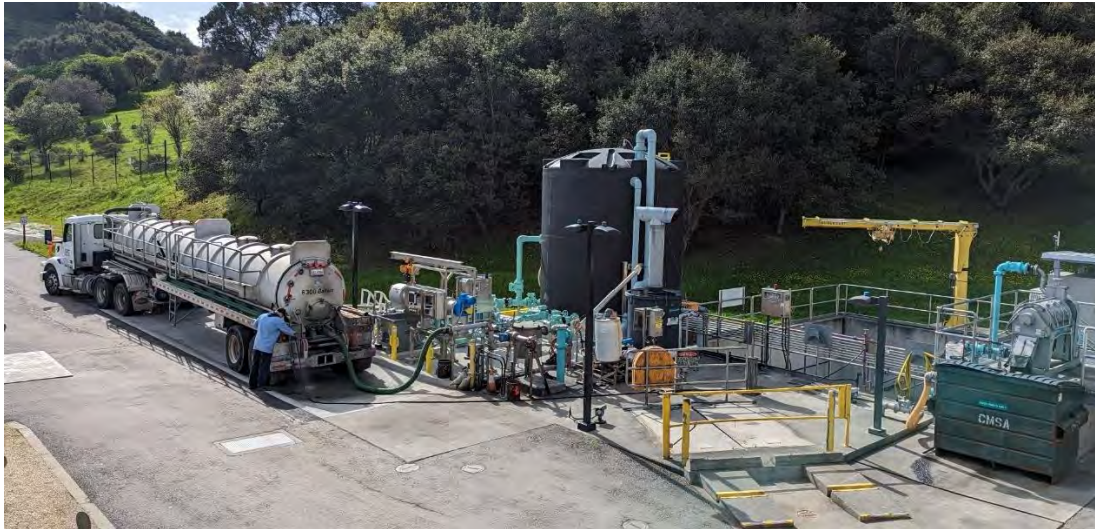
Figure 1: Truck contents being pumped through the new screening system and into the new Liquid Organic Waste Receiving Tank
